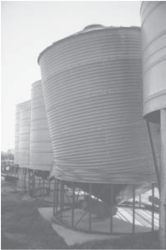
Figure 2. Silo distorted when outloading lupins.
