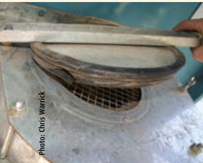
A weak seal: Replace broken seals to ensure sealable silos remain gas tight.
