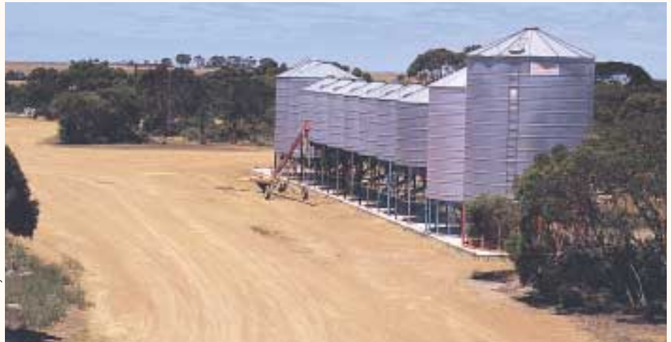
Silo aeration systems such as drying, cooling and maintenance can offer grain growers improved flexibility and marketing options at harvest time and provide more control over grain quality.
