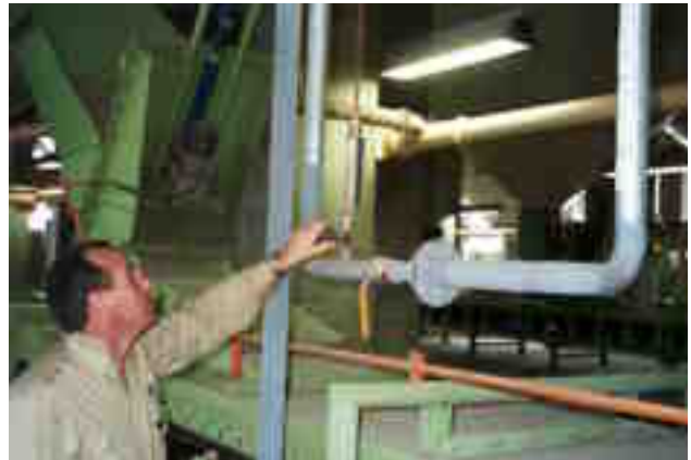
Figure 2. The under-bin pipeline system, with the Pest Control Officer adjusting the maintenance flow of nitrogen through the flow-meter.
