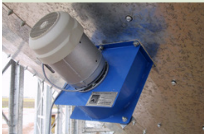
Aeration fan selected for cooling airflow outputs of 2–4 L/s/t
