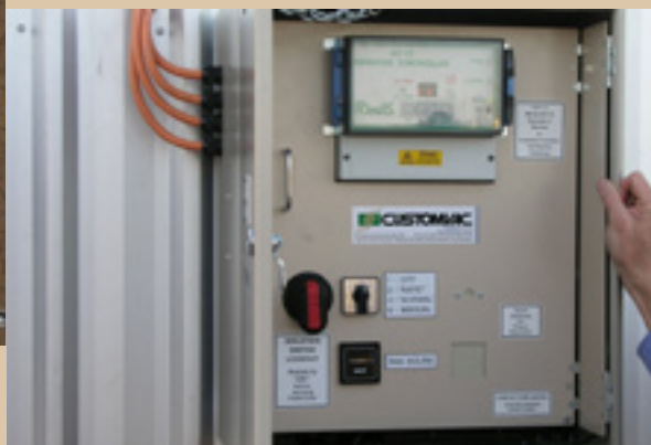
Example of an automatic aeration fan controller used to select optimum ambient temperature and humidity parameters for storage aeration fans
