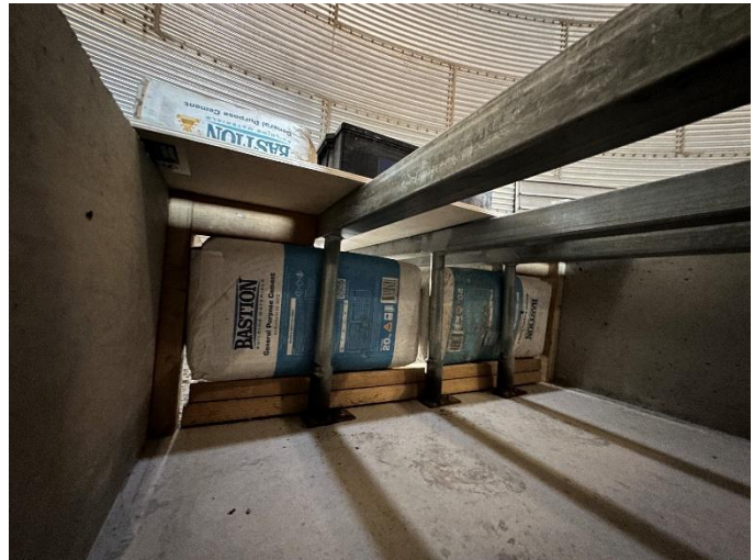
Figure 11: Bags of concrete and blocks of wood used to induce backpressure in the aeration trench of the axial flow fan.
