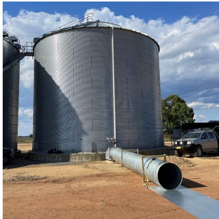
Image 1: 8m pipe made of sheet metal to measure airflow on an 800mm diameter aeration fan.
