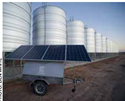
A power source trailer was custom-designed and positioned to maximise solar capture.
