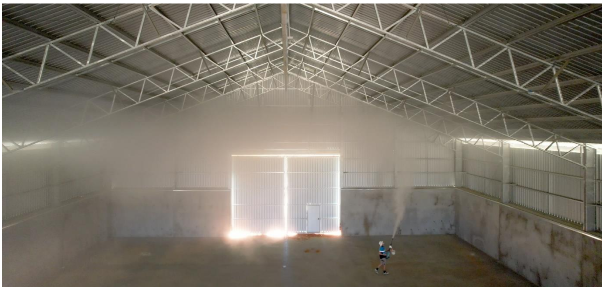
Application process, pointing the leaf blower at the roof while traversing the shed.
