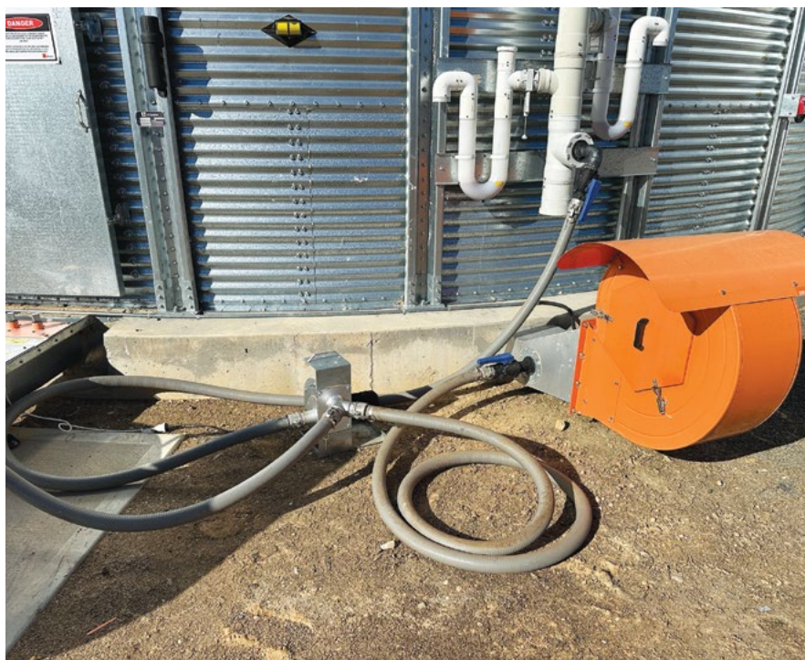
Photo 11: Recirculation can be achieved by placing phosphine in the silo and plumbing a small fan from the silo headspace to the aeration duct. (Source: Chris Warrick, Primary Business)
